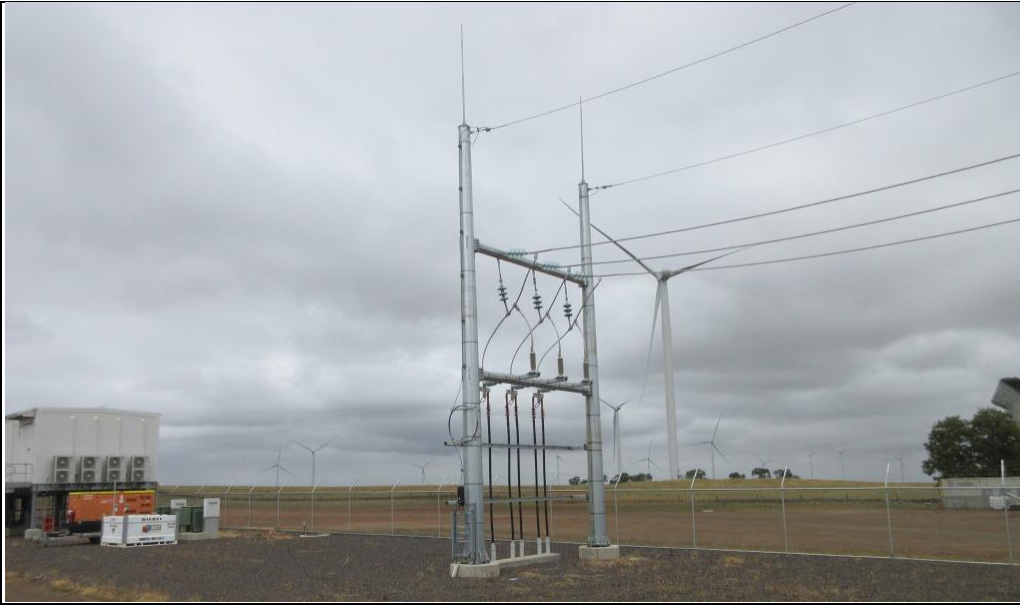
Plate 4.1 – Southern landing structure for 33kV line, at Western Substation
