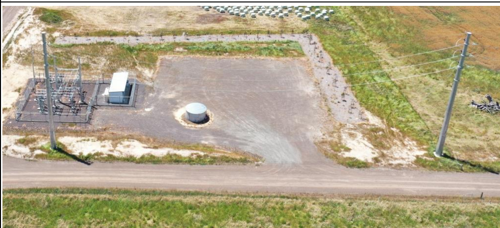
Plate 4.3 – Pole structures at Northern Transition Station, northern extent of line
